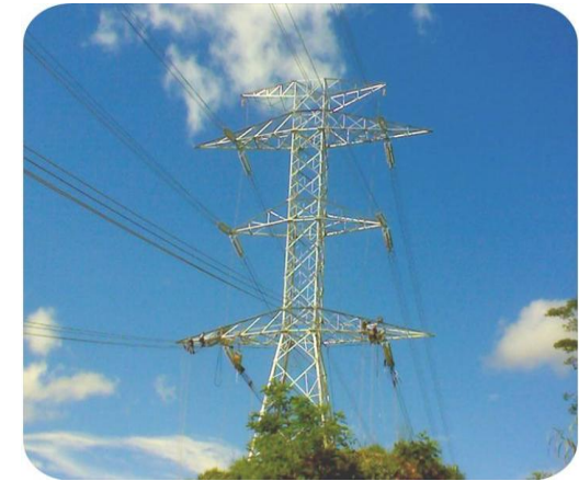
MURUM JUNCTION TRANSMISSION LINE 275KV EPC
